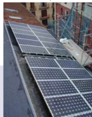
Roof mounted PV modules
