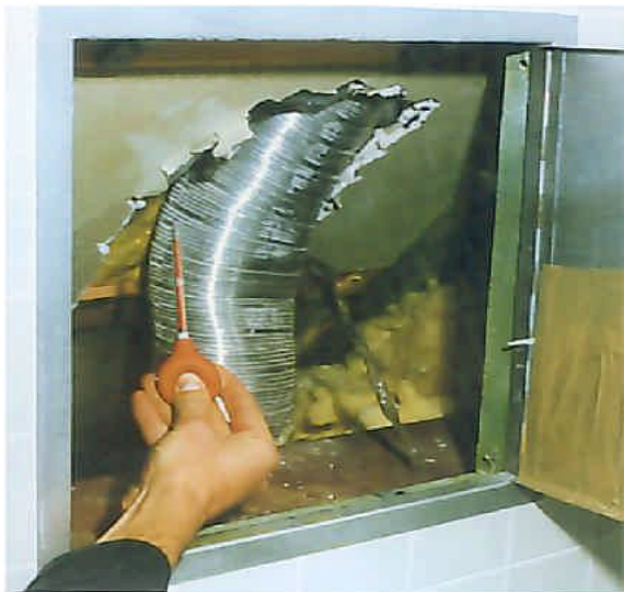
Fig. 4.1.4.: Ventilation pipe penetrates the function layer of the roof, massive leakage.
