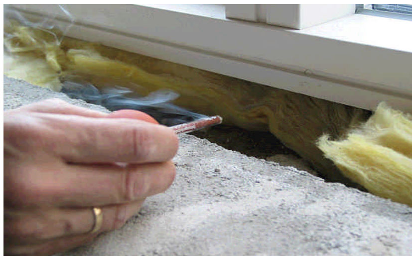
Fig. 8.2.2.: Example of registration of white smoke movement to trace cracks and crevices in combination with the blower door test.
