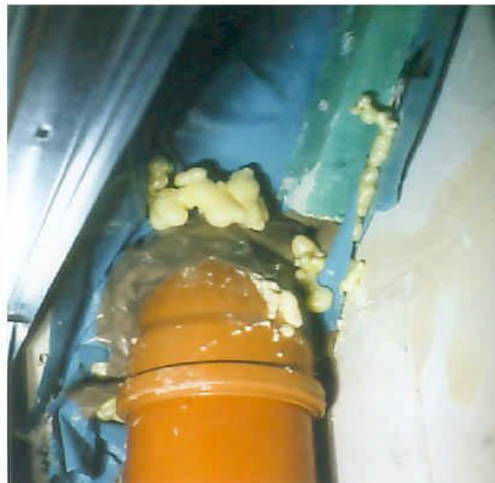
Fig. 4.1.5.: Pipe penetration – incorrect tightness concept in the planning phase. Because of the corner placing of the pipe a correct connection as regards workmanship
