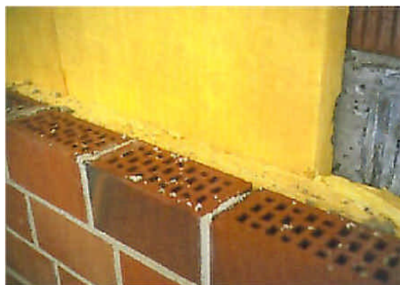
Fig. 1.1.1.2.: Securing of wind-tightness - brickwork with core insulation – here you see the layers from outside (front)to inside.
