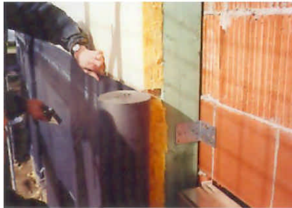
Fig. 1.1.2.1.: Securing of wind-tight - brickwork with insulation layer and ventilated coating on the back – here you see the order of the layers.
