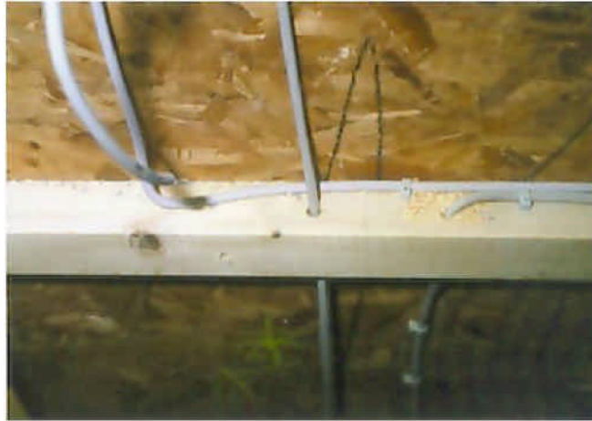
Fig. 1.2.3.1.: Mounting of electrical installation (e.g. for the electrical outlet) without reducing the air tightness using a thicker space for the wires.
