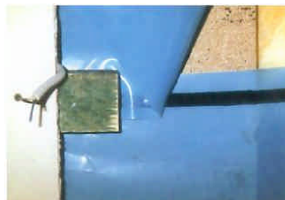
Fig. 2.1.1.6.: Installation of film assembling on a wooden plate. Overlap inserted sealing strip, mechanical securing (screwed on lists) hollow space for electrical installation and internal covering.
