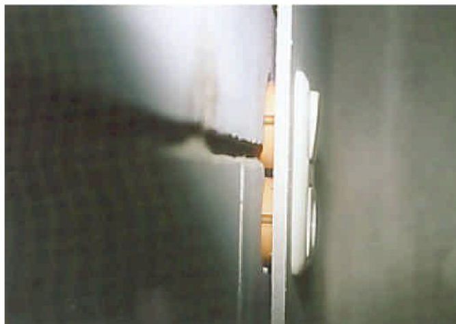
Fig. 1.2.1.1.: Dry-set cast, penetration point of the electrical outlet – in order to secure air tightness various measures are required.
