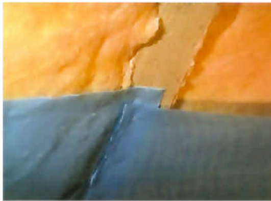
Fig. 2.1.1.1.: Sealing of the joining of the moisture barrier (length wise) on the rafter with overlap and fixed with clamps. Is not airtight.
