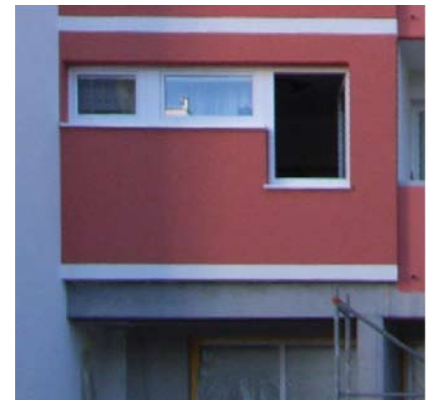
New situation around the entrance, after detection of thermal bridge with thermography
