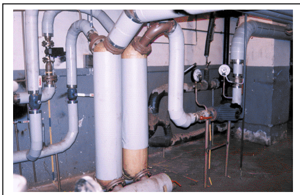
The heat exchanger at Przybylskiego 7 for Domestic Hot Water.
